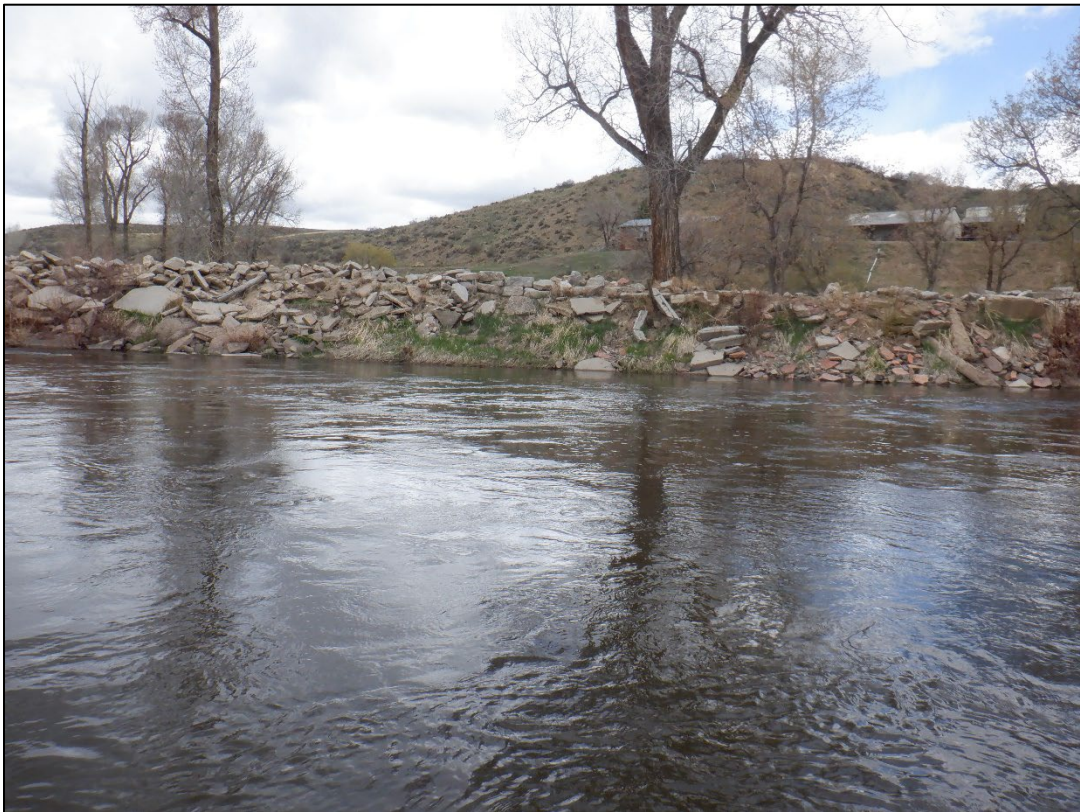
Figure A-8. Bank armoring with concrete.
