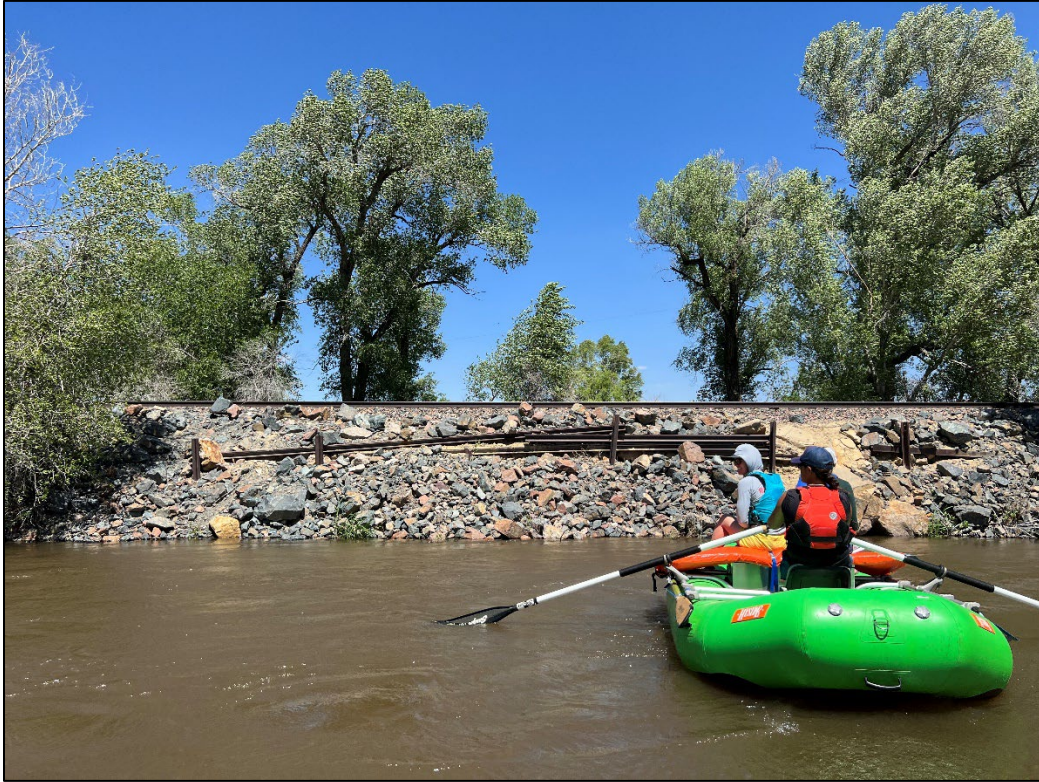
Figure A-5. Bank armoring to protect railroad infrastructure.
